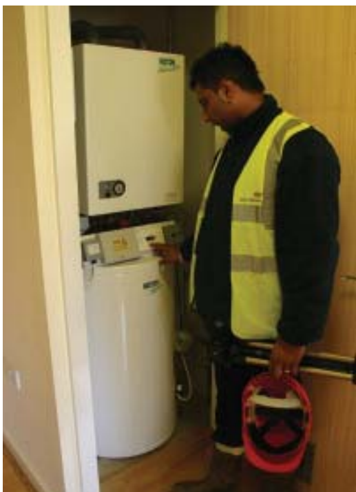
The boiler room at Grand Union Village (left).
